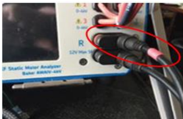
Figura 5.9 – Baker AWA-IV – Conexão Ponte Kelvin (MEGGER, 2019).
